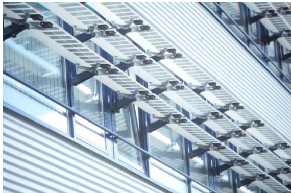
Fig. 11: PV Shading System, Eschweiler, Germany
